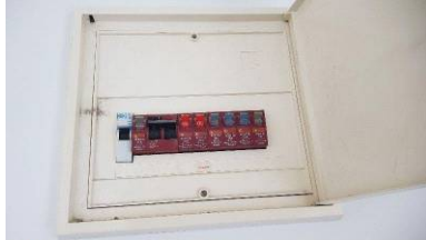
Fuse board to interior
