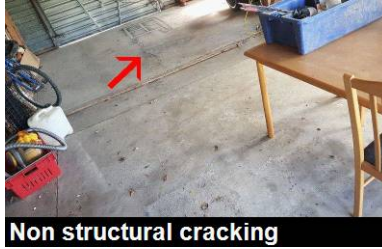
Non structural cracking
