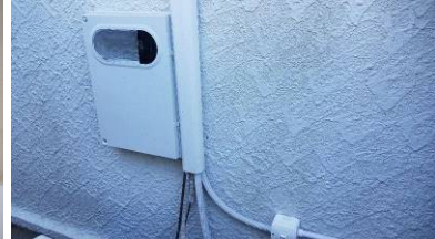
Meter board to exterior
