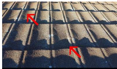
Significant aging to roof surface
