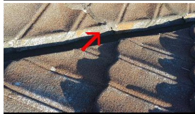
Rusting to valley tiles
