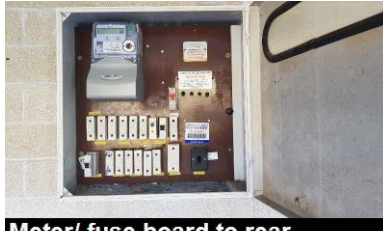
Meter/ fuse board to rear exterior
