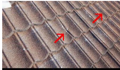
Dent damaged tiles
