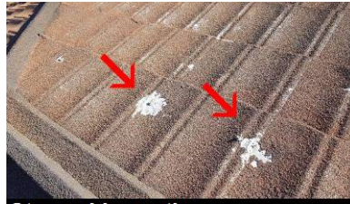
Stone chip coating deteriorating
