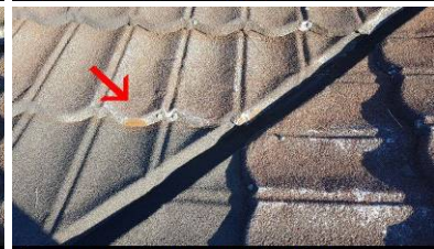
Some surface rust to tiles
