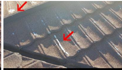
Significant wear to tiles
