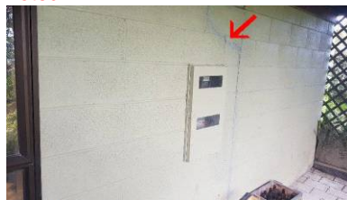
Meter board to exterior, cracks evident
