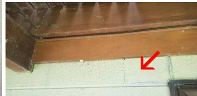
Cracking sesaled to blockwork
