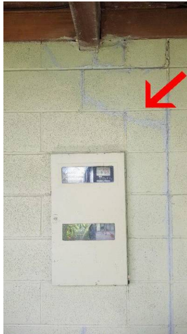
Cracking moving towards expansion area
