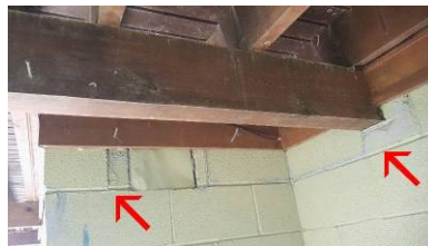
Cracking to bondbeam block work
