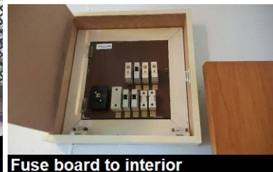
Fuse board to interior
